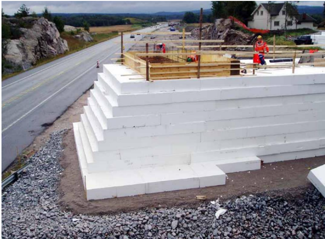
Figure 3.5: Use of EPS in an interim bridge over E6 at Gimsøyvegen. Photo: Tor Helge Johansen.
