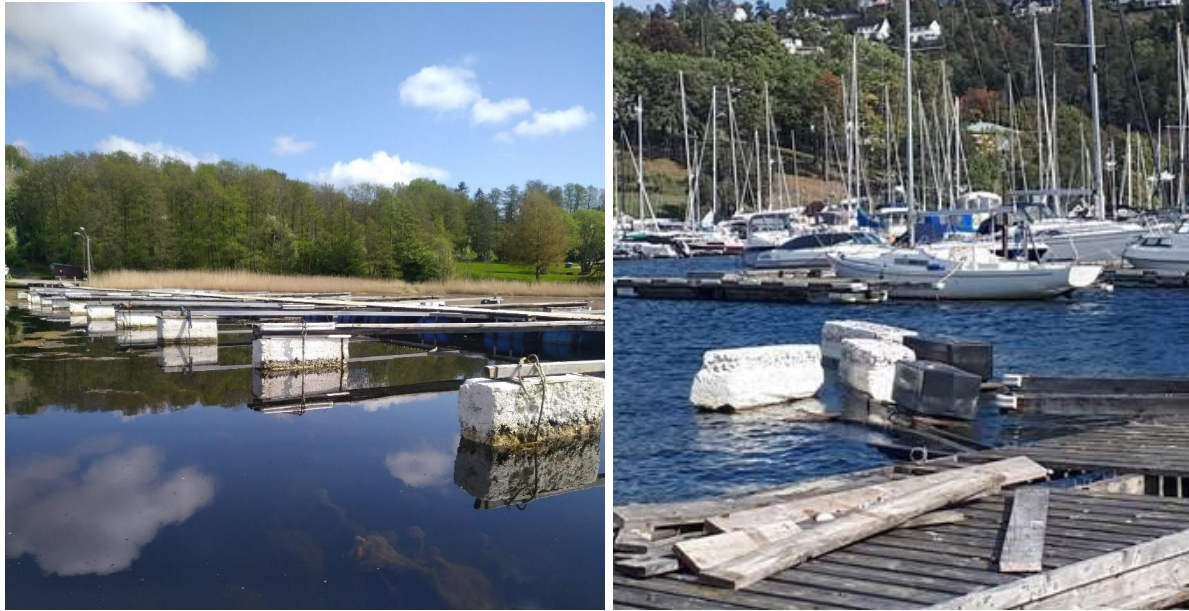
Figure 3.10: Used EPS blocks used as pontoons. Photo: Oslofjorden friluftsråd. -Right: Pontoons torn during heavy weather.
